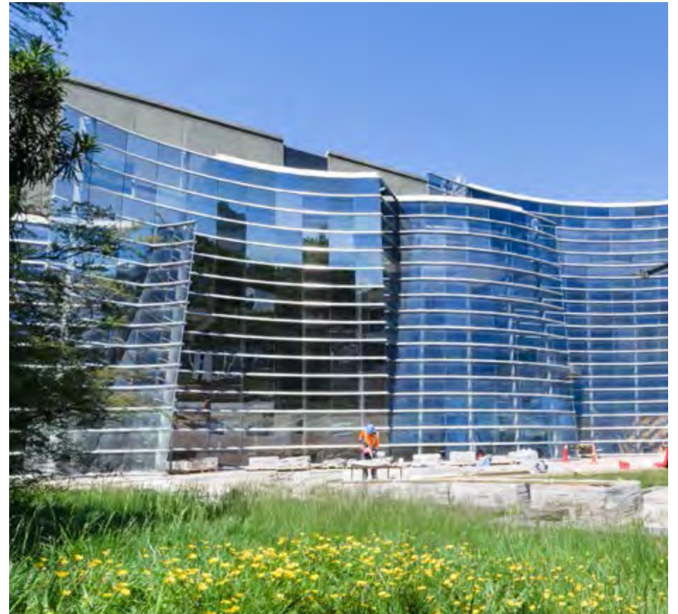
Counting down: Christchurch Art Gallery moves closer to re-opening as earthquake strengthening work continues.
