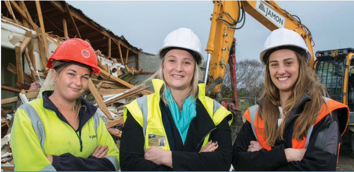
(From left) Bianca O'Neill, Kate Dirkwager and Victoria Esson enjoy working in the male-dominated construction industry.
