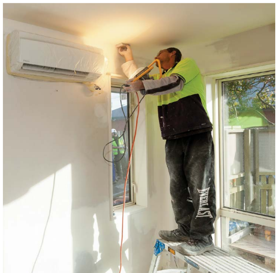
A Housing New Zealand contractor carries out extensive repairs inside an earthquake-damaged property.
