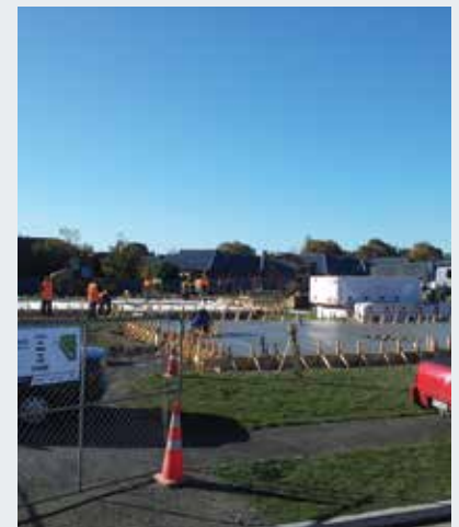
Foundations being prepared at the new Rangers Park housing development in Linwood.
