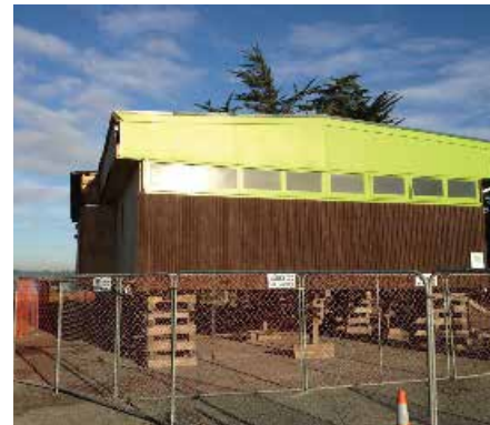
The former QEII Preschool building, which will become the transitional community centre, sits on blocks while foundations are built.
