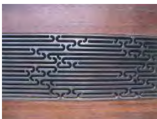
Government House Floor Vents
