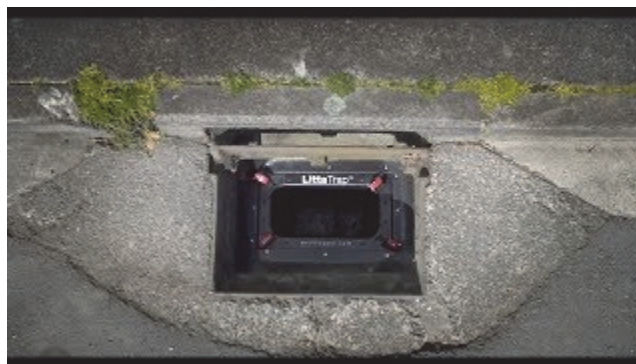
Figure 53 The LittaTrap in place to prevent plastic and other litter entering the waterways through the drainage system
