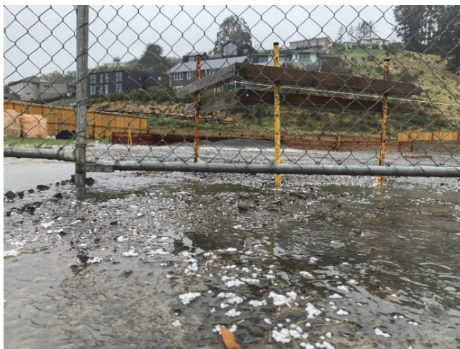
Figure 15 Expanded polystyrene from a construction site entering the waterways.
